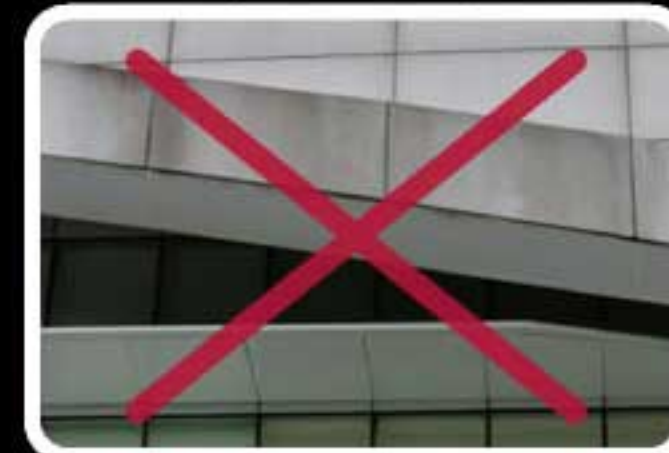
Streaking (Silicone Sealant)
