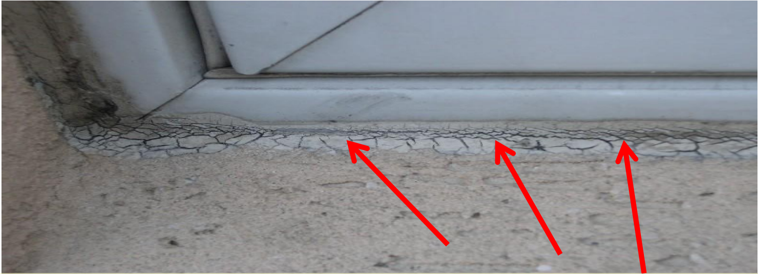
Cracked PU(Polyurethane) Sealant (Window Perimeter Joint)
